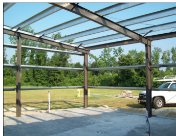
Construction on the 900 sq. ft. addition started in the spring and was completed in November 2009.
